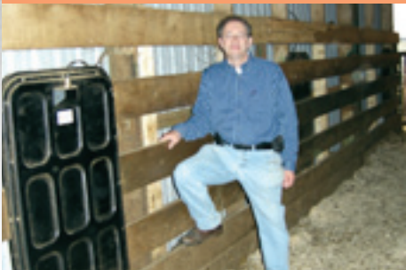
Destron Fearing's Paul Laronde installed this wide-alley reader with antenna, which captures RFID numbers. This allows animals to move at the speed of commerce.
